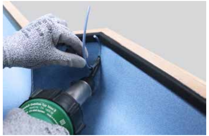
2. Thread the weldrod through the nozzle and weld the joint starting from the top.
