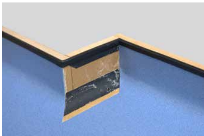
2. Fit the flooring to the back wall. Trim off the excess height and cut in the internal mitre. Bring this cut down the corner until it reaches a minimum of 20mm from the bottom edge of the cove former. Continue the cut parallel to the cove former until it has joined up with the external mitre.
