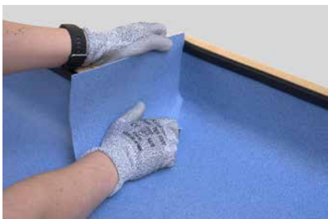
3. Using a pre-adhered section of flooring roughly cut to the size of the infill section, fit tightly into the internal mitre before adhering the section to the wall and cove former.
